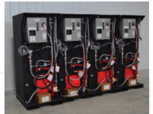
Fire protection for Mobile Housing Units.
